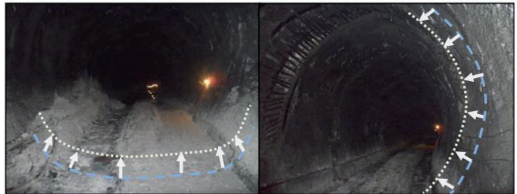
Figure 1. Squeezing at Chameliya Hydroelectric Project Headrace Tunnel (CHEP) (Basnet, 2013)
