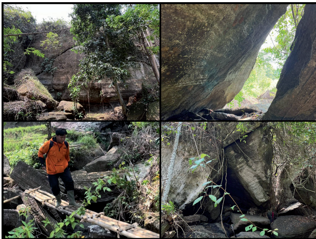
Figure 5. Geosite condition of Taman Batu Sarongge, highlighting potential hazards such as a narrow wooden bridge without handrails, slippery moss-covered rocks, and weathered rocks
