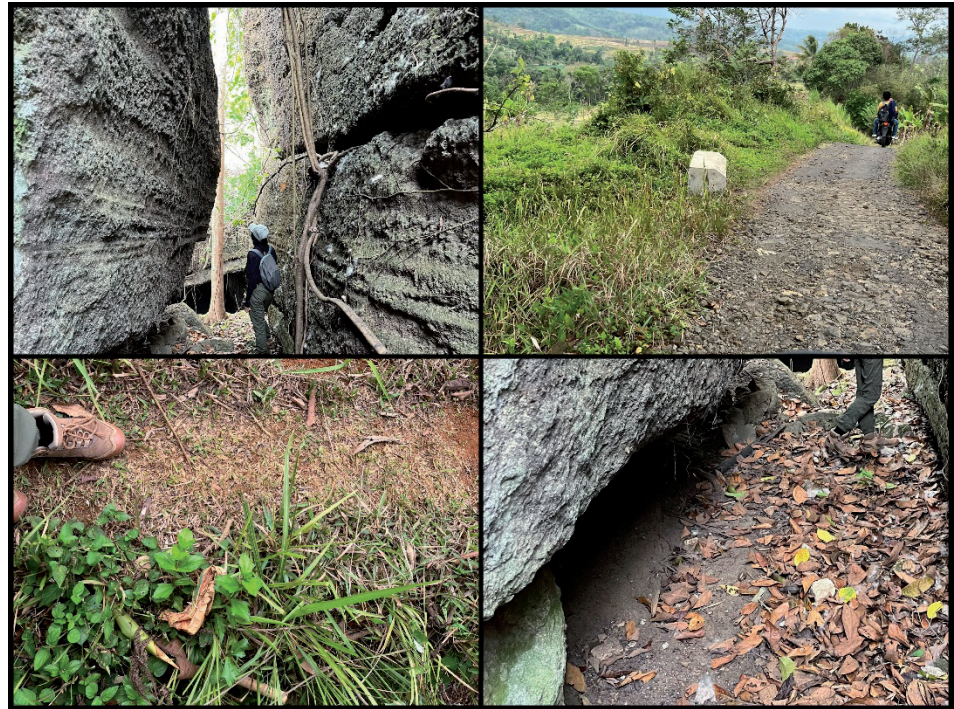
Figure 4. Geosite condition of Taman Batu Cukcrukan, highlighting potential hazards such as uneven roads, narrow paths, dry leaves covering trails, and weathered rocks.
