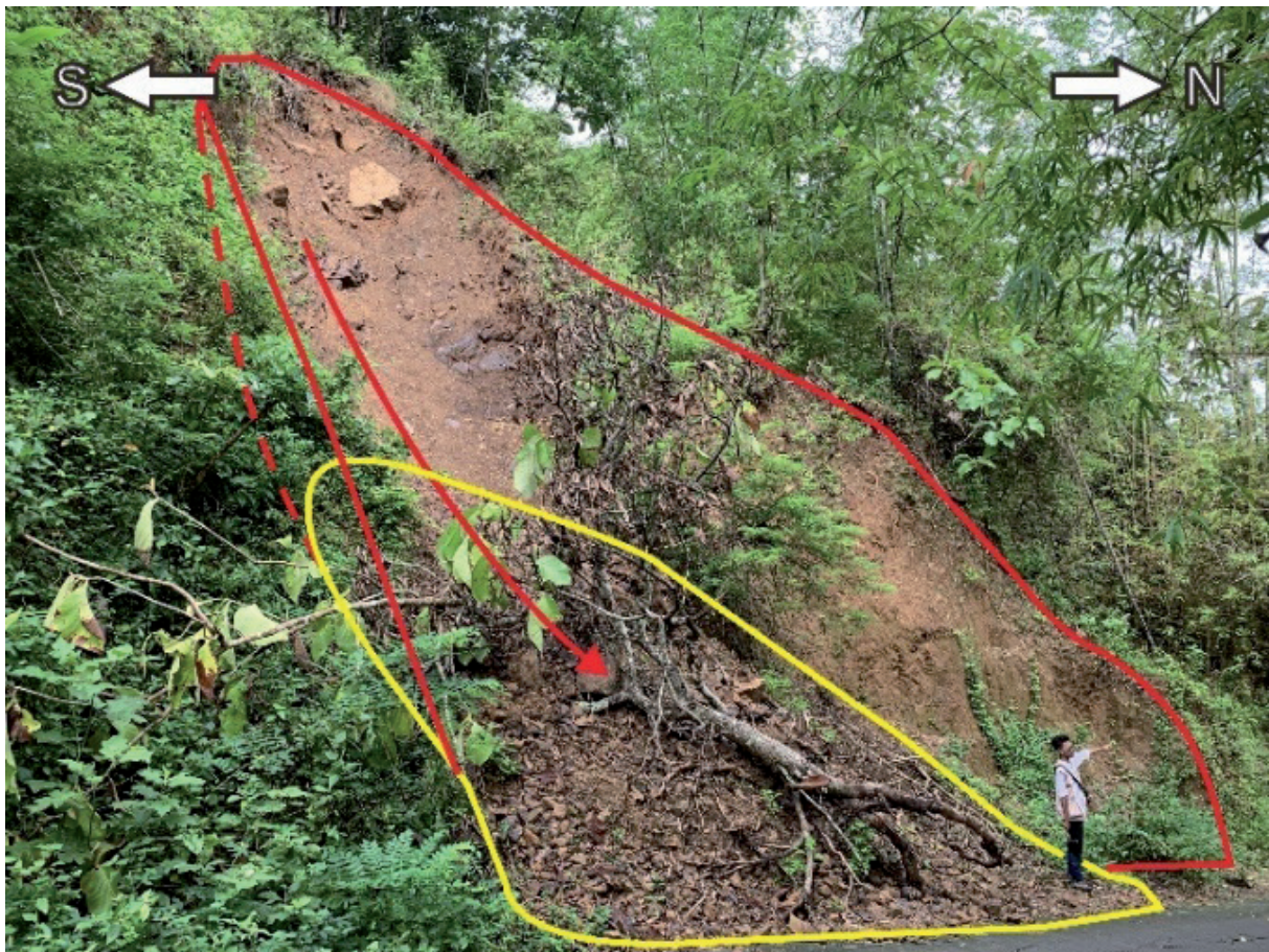
Figure 9. Landslide evidence in the slope angle class of 16°-35°
